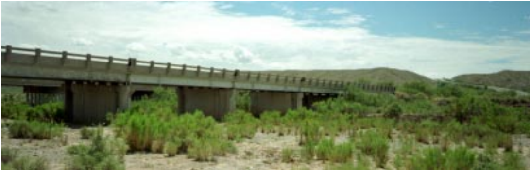
Figure 7.1: A side view of the Alamosa Canyon Bridge (Courtesy of the Los Alamos National Laboratory)
